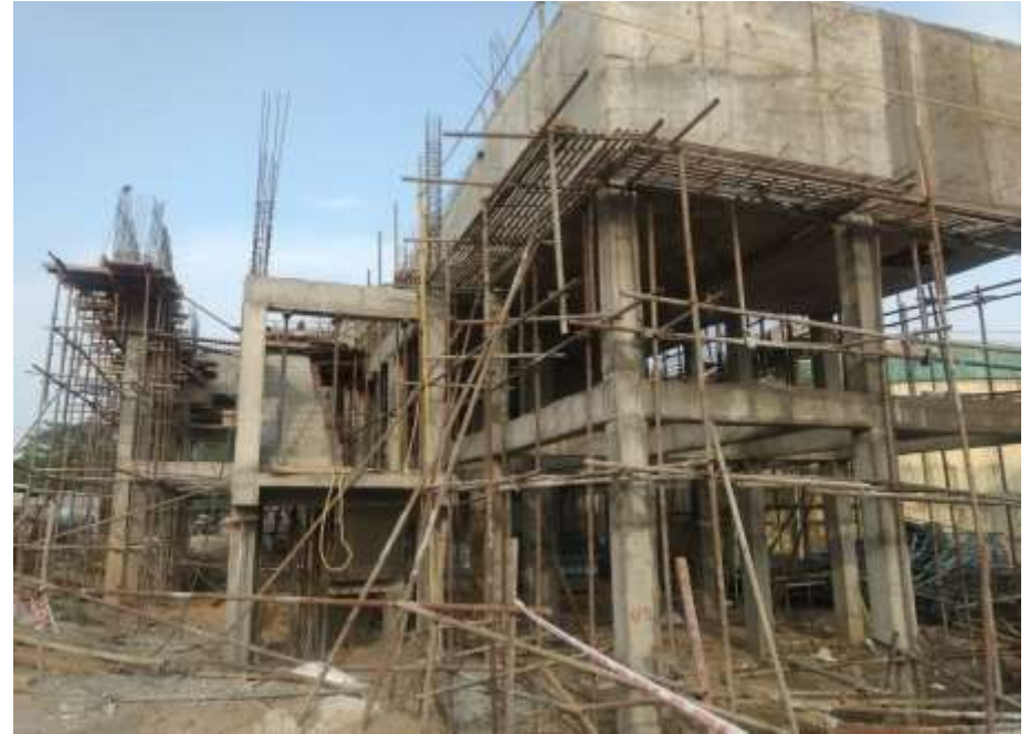
Saidpur STP (60 MLD), Patna
