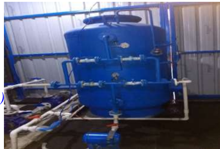
Karnaprayag – STP - Filter Vessel
