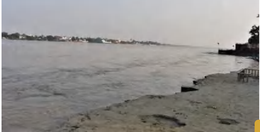
Erosion Prone Bank of Gandak River
