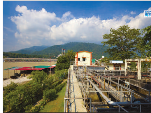
Rishikesh (Swargashram) 3 MLD NJK (STP)
