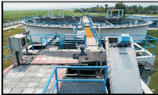
Operational 12 MLD Sahibganj NJK (STP)
