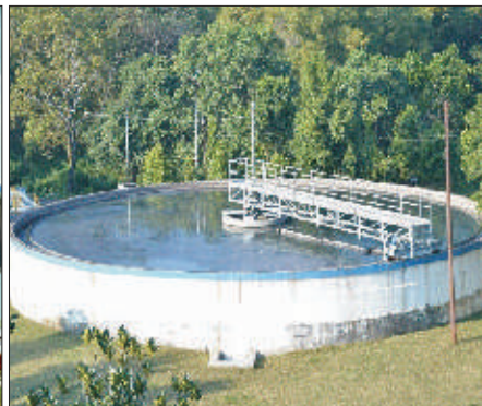
Kalyani 21 MLD NJK (STP)
