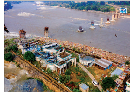
Srinagar 3.5 MLD NJK (STP)
