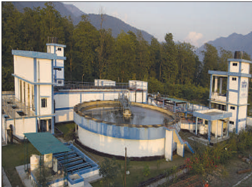
Chorpani, Muni Ki Reti 5 MLD NJK (STP)
