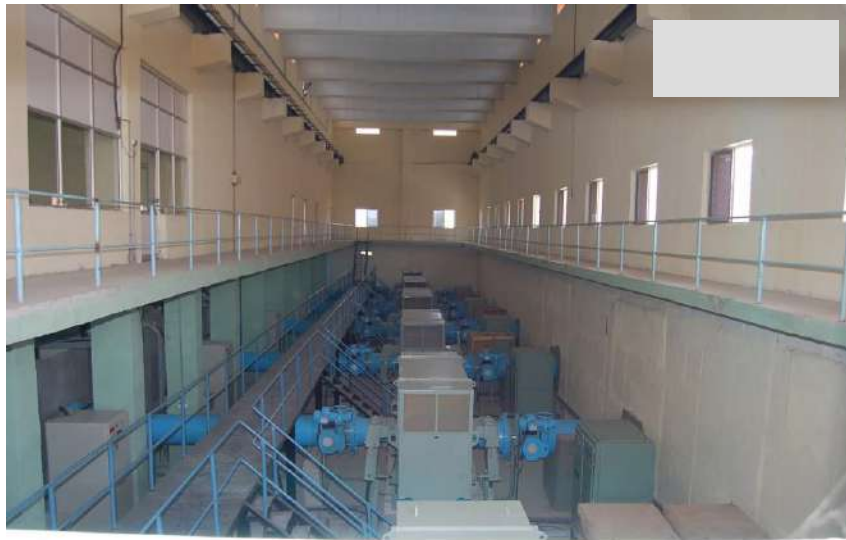
Pumping Installation - Godakondla
